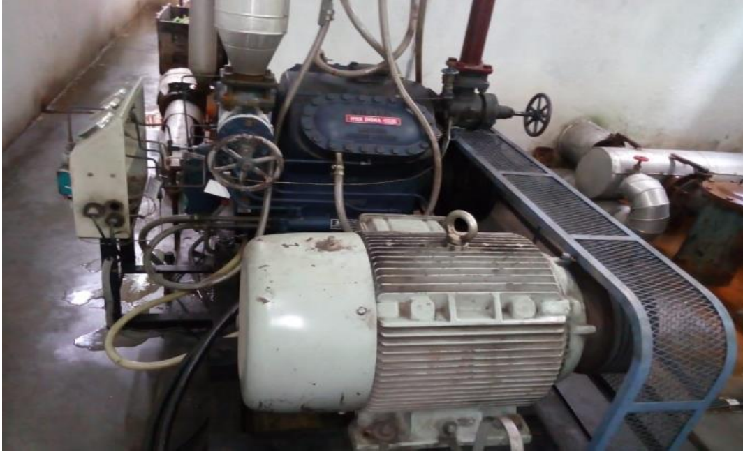
Image 3: Chiller compressor at Sikkim Dairy Cluster
